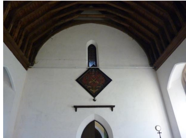
West end of nave with window at first floor level into tower
